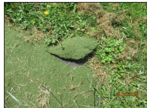
(Damaged artificial turf)
