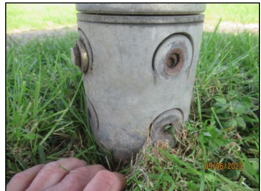
(Broken studs at ground fixing)
