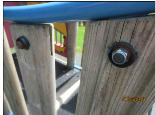
(Broken bolt cover caps)
