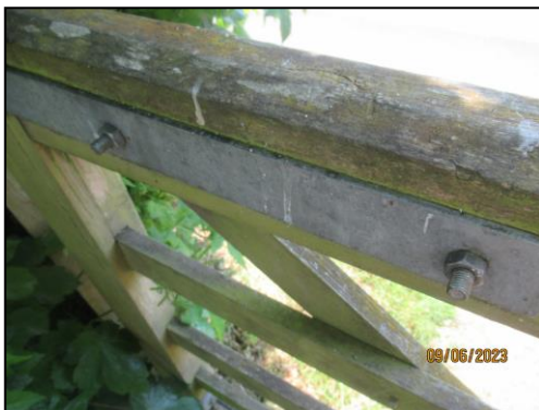
(Excess bolt thread at gate at skate park)
