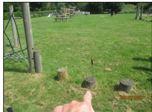
(Rotten step post)
