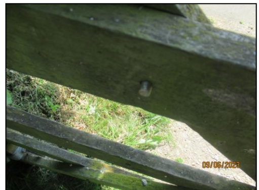
(Missing nut on bolt at gate at skate park)
