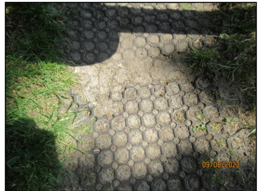
(Damaged grass mat)
