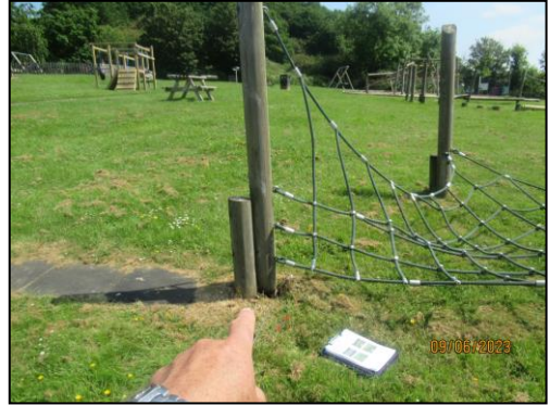
(Location of rotten post on net climber)
