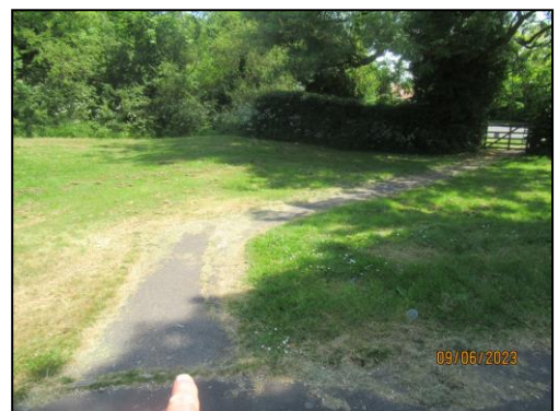
(Poor condition path)
