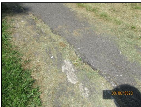
(Poor condition path)
