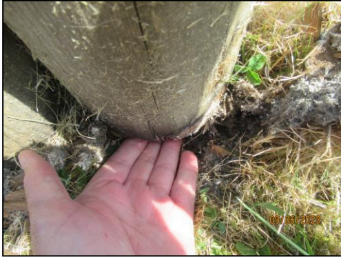
(Rotten post on net climber)
